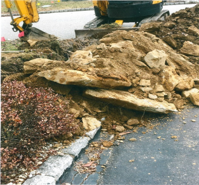
30 Seasons Glen: Existing service installation with no controlled back fill and large rocks against the service line. 2
